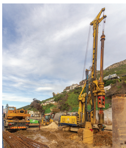
(Above): Powerful rotary piling rigs were deployed to install the main piles to support the building, penetrating the underlying boulders.
