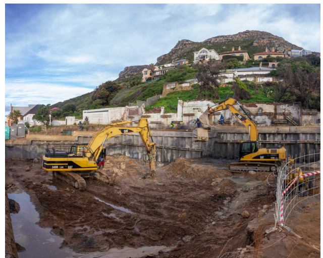
(Above): The new soldier piles and capping beam integrating with the newly-bolstered existing retaining structure.
